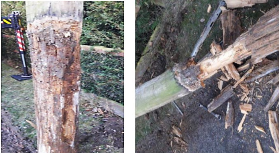
SEVERE POLE DECAY BELOW THE GROUND LINE
