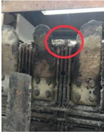
FAILED LV BOARD DUE TO THE LOOSE CONNECTIONS. THERMAL INSPECTION AND CONDITION ASSESSMENT MAY HAVE ENABLED EARLY DETECTION.
