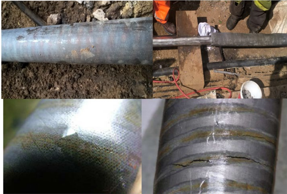
Crack in Lead Sheath caused by Crystallisation of the lead
